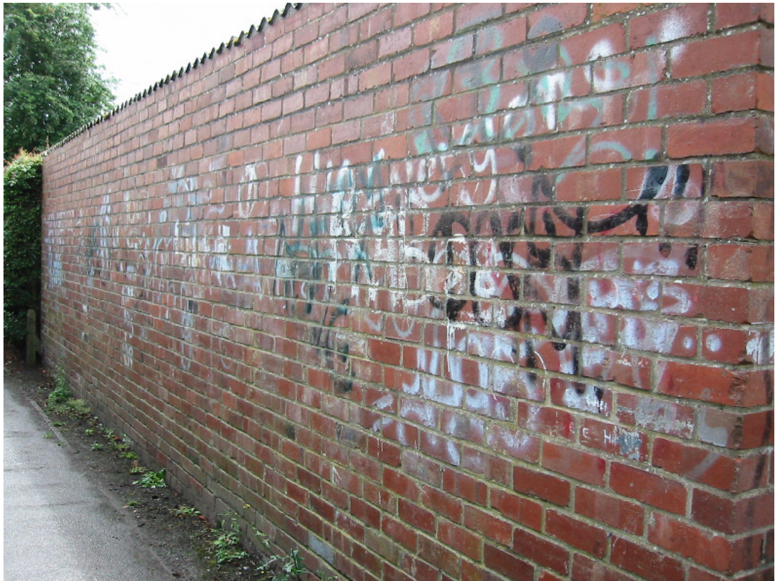
Fig. 3: Graffiti along the wall of the snicket (rear shed wall of 81 Beckfield Lane)
